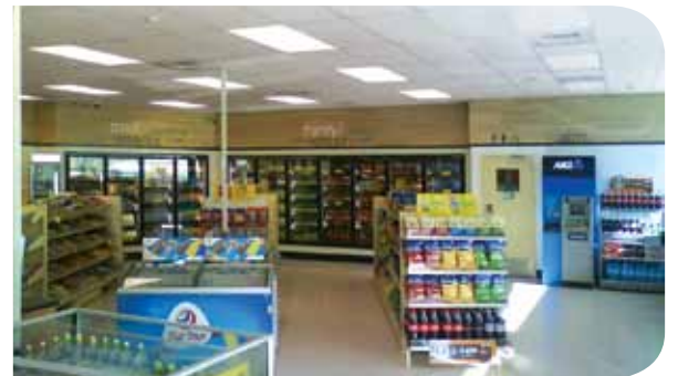
Daylight dimming in BP Connect Rosedale, Albany. The row of fittings to the top right of the photo is dimmed completely, taking advantage of natural light near the front of the outlet (on the right of the photograph).
