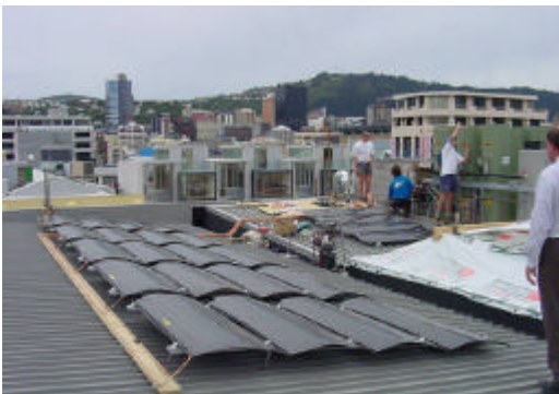
Enviro panels for the heat pump hot water units at YHA, Wellington
